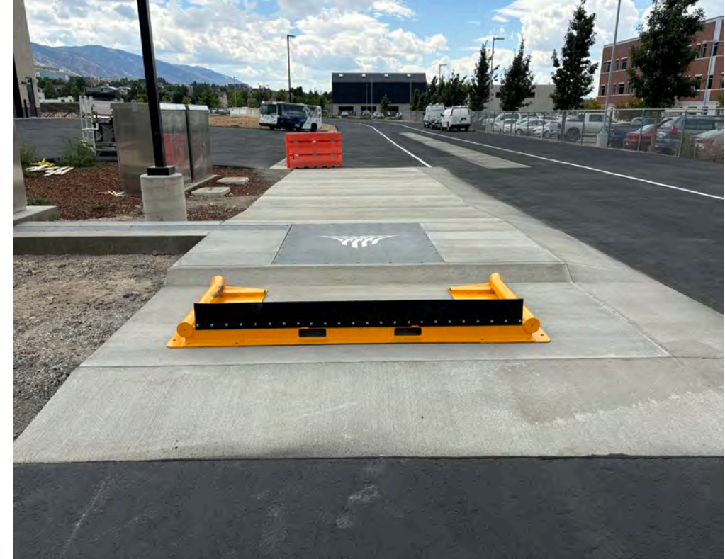
Megawatt Charger In-road Charger
