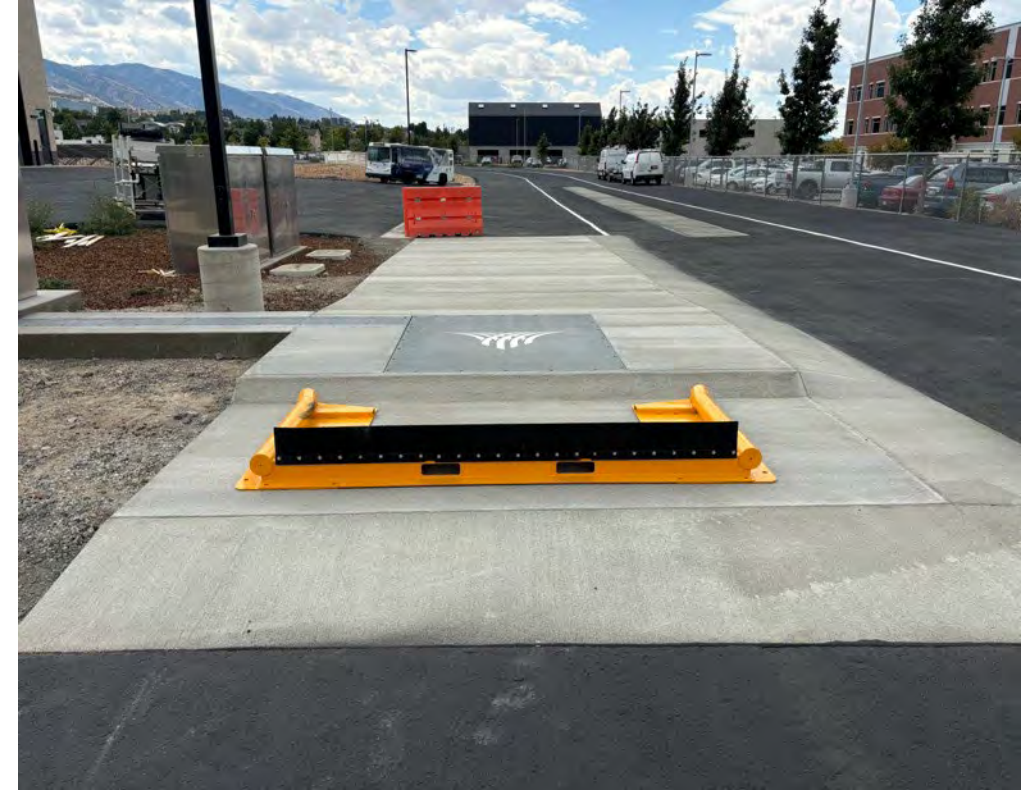
Megawatt Charger In-road Charger
